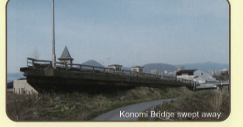
Hot mudflow swept Konomi Bridge (which used to span National Route 230) a distance of 100 m from its original location.
