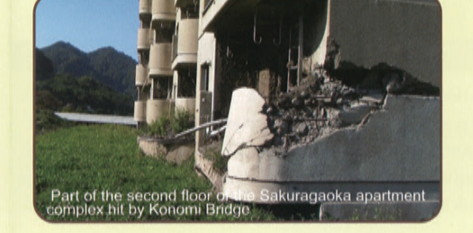
The first floor of the Sakuragaoka apartment complex was buried in gushing hot mudflow from the eruption in 2000, and the second floor was scarred by Konomi Bridge as the photo shows.
